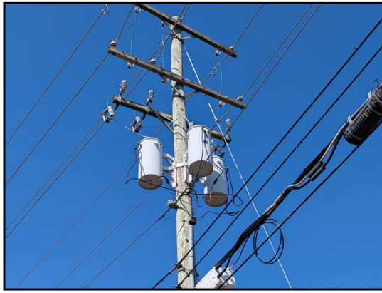
Photo 9 - Typical view of pole-mounted transformers
