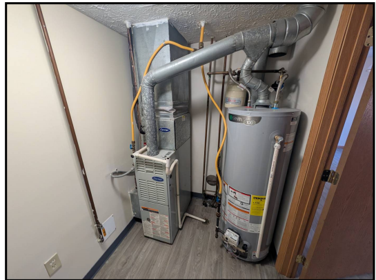
Photo 28 - Representative view of unit utility closets
