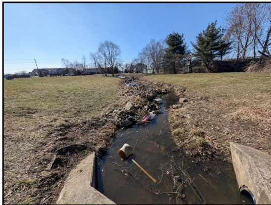
Photo 11 - View of the drainage system to the retention pond
