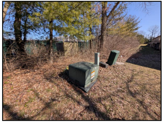
Photo 14 - Representative view of pad-mounted transformers
