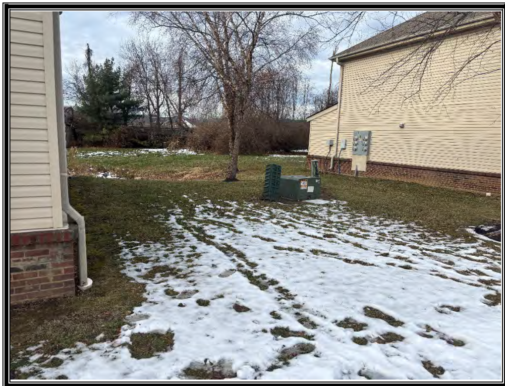
Photo 4: Representative view of a pad-mounted electrical transformer on the property.
