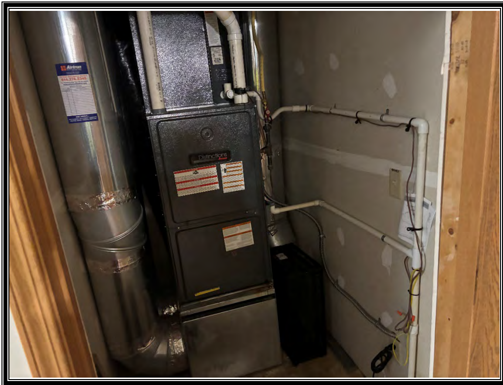
Photo 7: View of the furnace in the leasing office.
